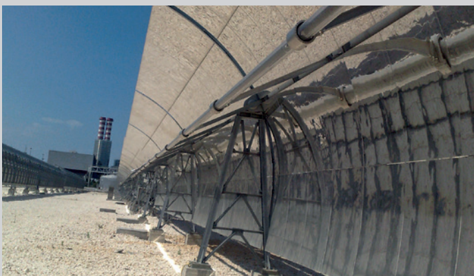
Archimede project, Syracuse, Italy A hydraulic motion system moves and controls the huge parabolic mirrors to capture the sun's rays at the solar field
