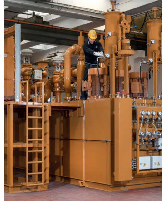
Steam turbines - lubrication
